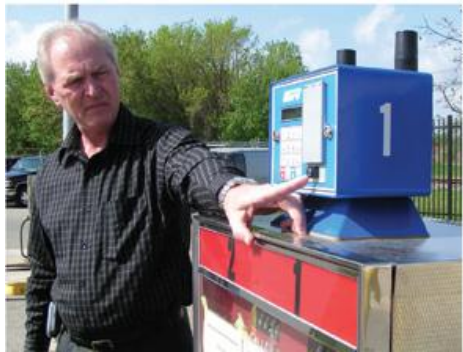
Bill VandenBrook, Madison's motor equipment superintendent, points out the pump module, which is part of the Automated Fuel Management System.
